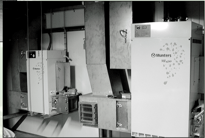
The completed dehumidification unit.
