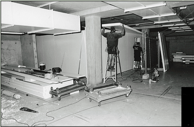
Construction of the State Library's new film vaults. Shown is the installation of the panelling.
