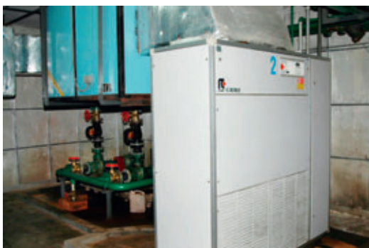
4. Air-conditioning system to keep the constant temperature and humidity.
