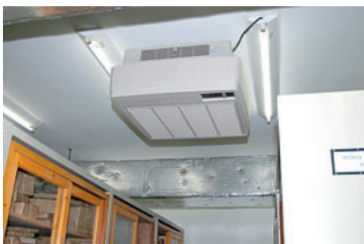
5. Air purification facility installed in the special collection stacks.
