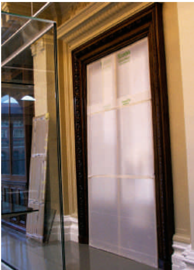
3. Example of dust protection to manage the effects of building activities. Photography by V. Blyth. © V&A images
